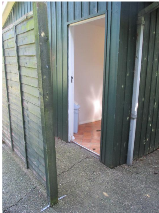
Entrance to male toilets (79cm width). The male cubicle has an outward opening door. There is no handrail and no emergency cord
