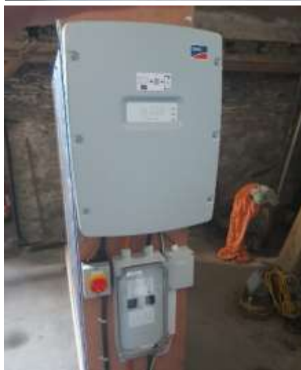
New battery bank & inverter
